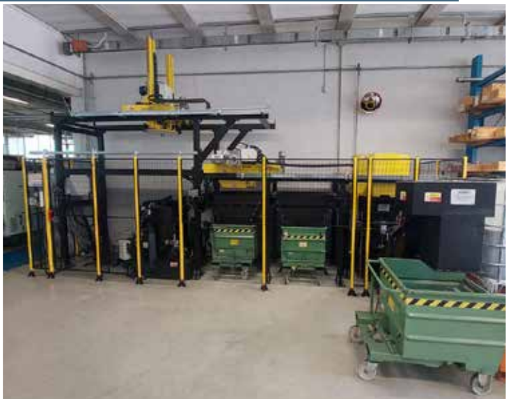
Plant with three discharge stations for steel, brass and stainless steel
