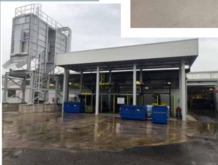
Plant equipped with centrifuge for aluminum and brass with silos
